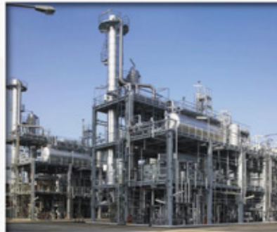
Fire Fighting Pipeline of Moroccan Chemical Plant
